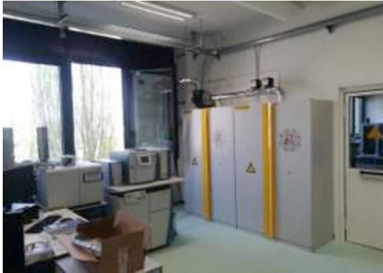
IRMS Gas cabinet
